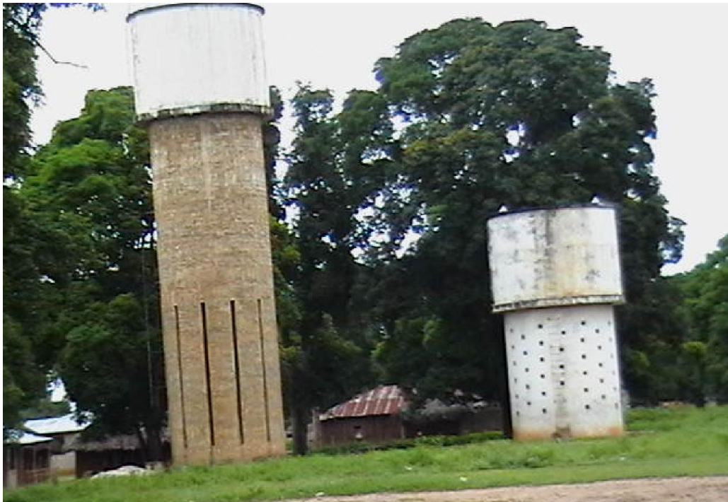
Figure 2: Two water tanks at Ikwiriri
